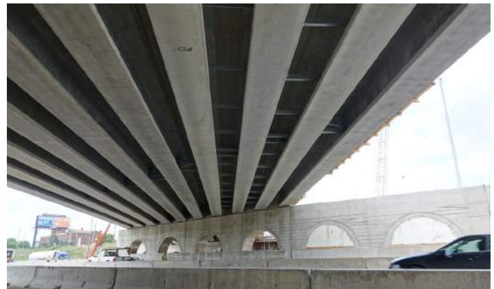
Concrete beams under the east half of the Gratiot Avenue bridge constructed in 2018.
