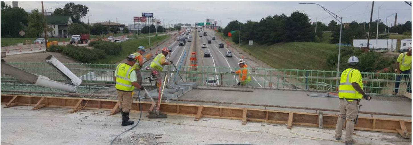
A construction team creates a new sidewalk at the Chene Street bridge.
