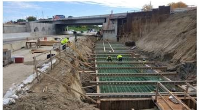
At the Gratiot Avenue Bridge, getting ready for the next concrete pour.
