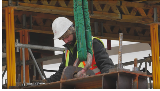
Diego Bustamante, a member of the Second Avenue construction team, at work.
