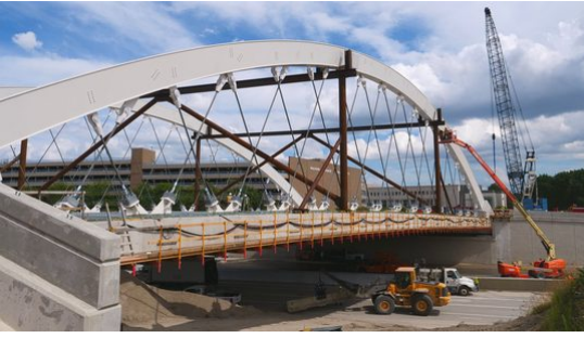
Progress on the Second Avenue bridge is driven by a diverse team.
